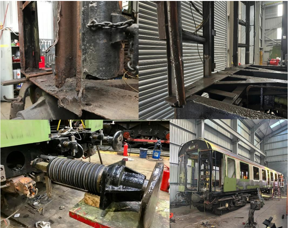
Clockwise from top left showing progress on FO 3112, representative of the magnitude of work being carried out on many of our mk1 coaches: Crash pillar corrosion before repair, repaired crash pillars and new sole plate, fully overhauled buffers & draw gear being fitted, and general view of repairs with all windows and ends exposed to rectify corrosion where required.
